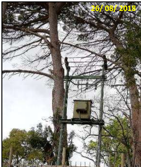
Figure 20: The exposed transformer box at Veels-te-Ver.
